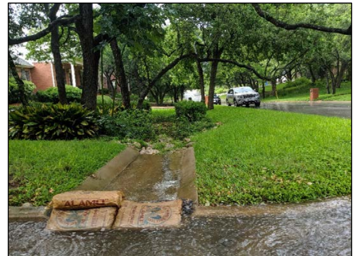
200 Wallis Drive, during rain event. 06/06/2019
