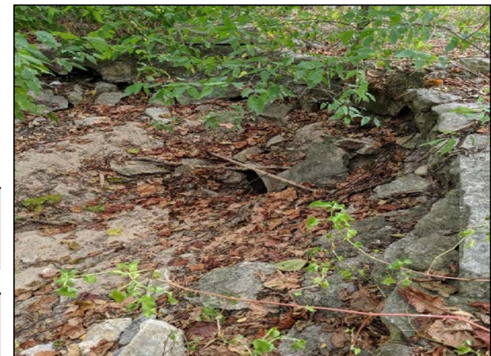
Half buried culvert at Rollingwood Drive. 09/11/2019
