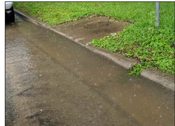
Pond inlet during rain event. 06/06/2019
