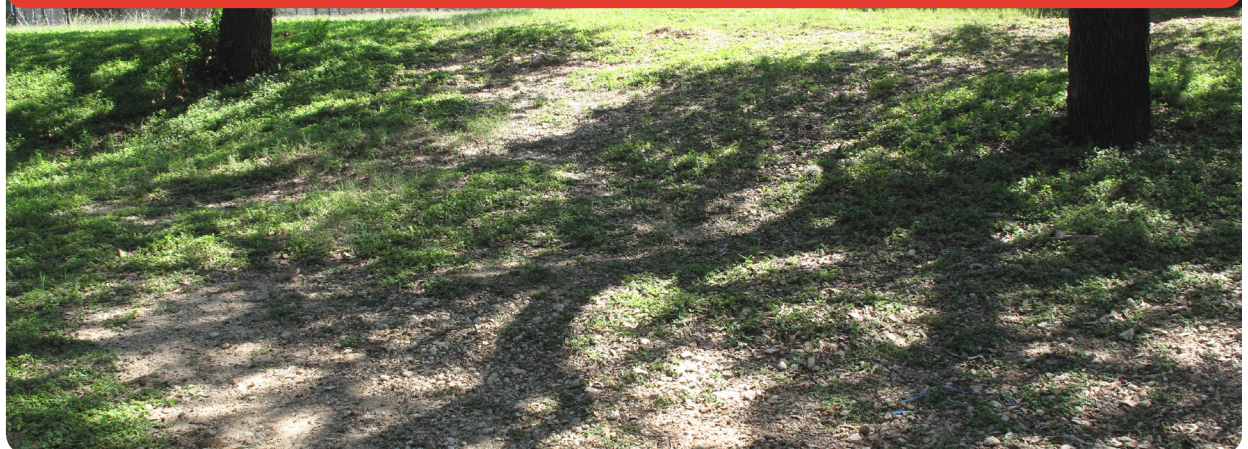
on going drainage issues of erosions of the bluff and hillside
